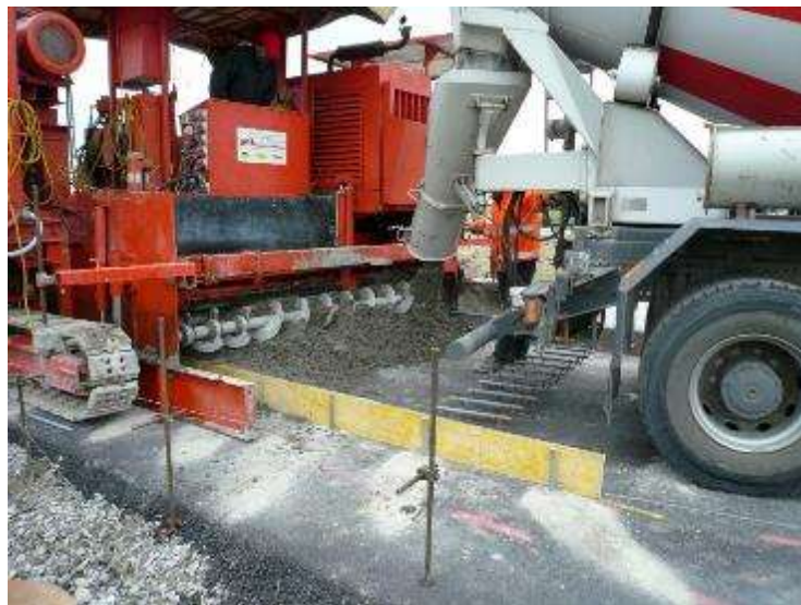
Figure 2: Paving the fresh concrete using a concrete finisher over the 5 cm thick asphalt base at the roundabout (Hrapović 2, 2020, S. 265)
