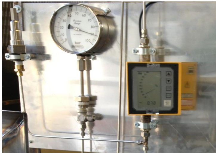
Figure 2: Pressure Gauge and GTMX flow Meter
