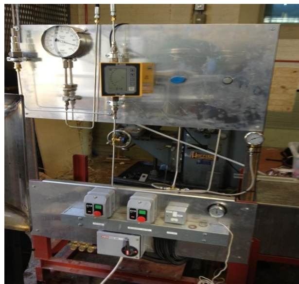
Figure 5: Injector System Control Panel
