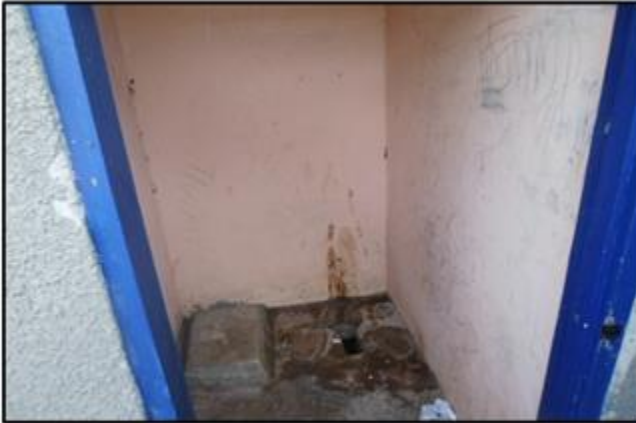
Filthy School Toilet (Faecal matter scattered all over the Toilet Floor.)
