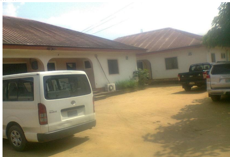
Plate I. Dark-Black Deposit on Colored Roofs in a Housing Estate in Uyo Town
