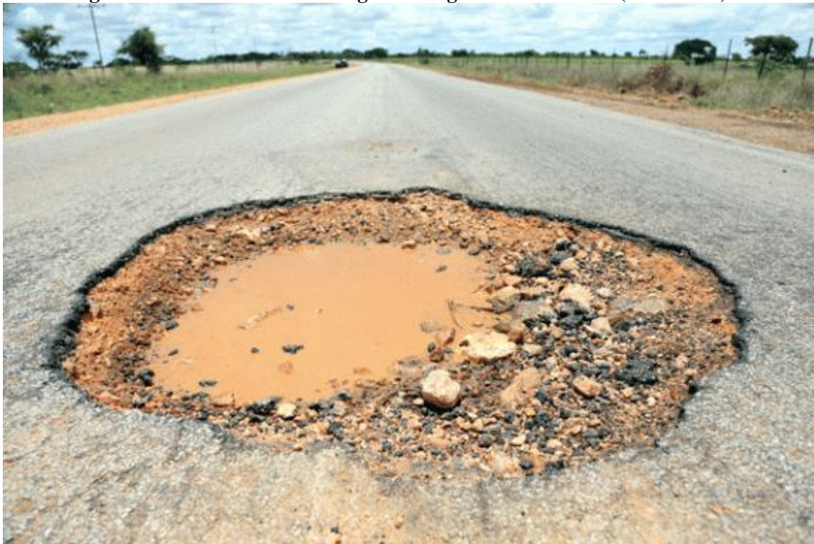
Figure 1: Pothole identified along Beitbridge-Chirundu Road (Zimbabwe)
