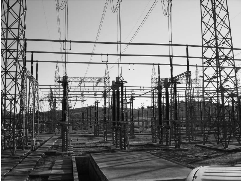
Figure 2. Switchyard of measured iron – steel facility
