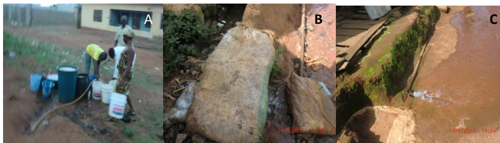
Figure 5. (A) Improper connection at GRA, Wukari, (B) Leakage covered garbage sack at Kaka Qtrs, Gembu, (C) Leakage along network at Mansur Qtrs, Gembu
