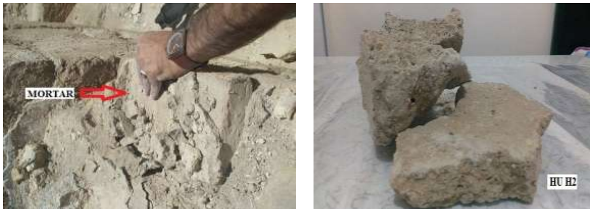
Figure 8. Mortar sample numbered HU H2 which was taken from Harran University
