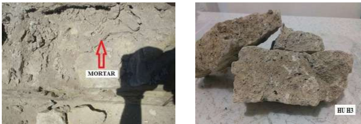
Figure 9. Mortar sample numbered HU H3 which was taken from Harran University
